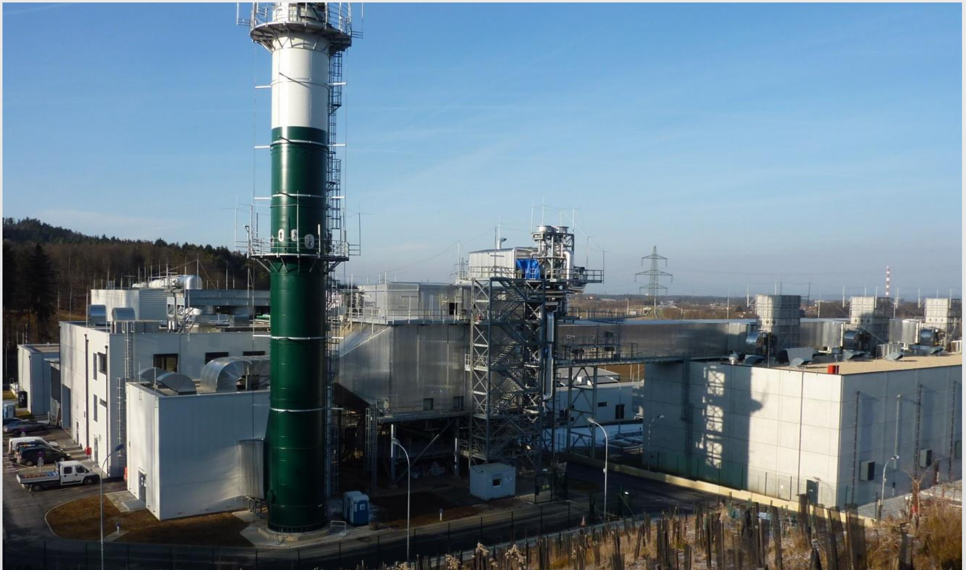
Ecoflow at OMV, Austria - Turn key project including civil works, waste heat recovery plant for power generation
