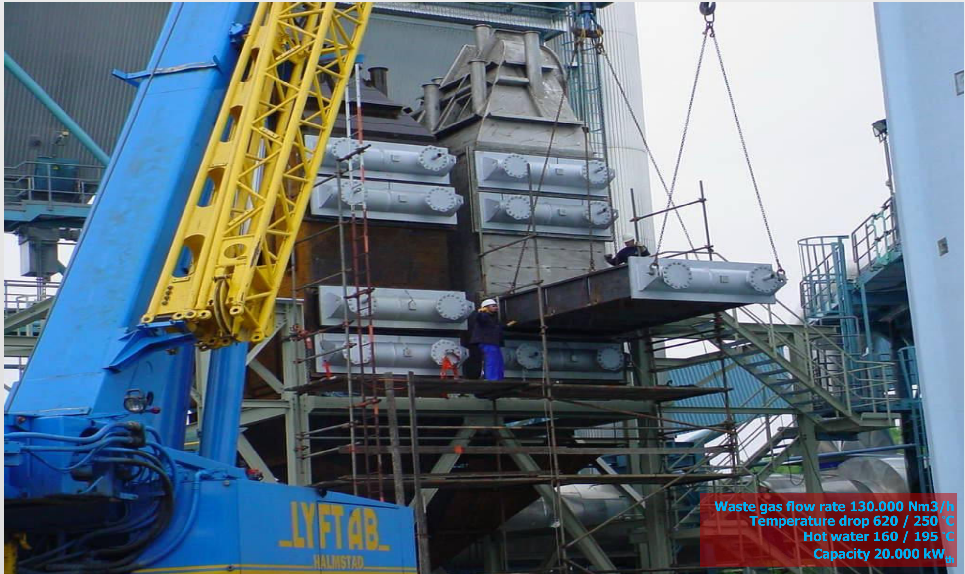
Ecoflow in glass industry waste heat recovery from flat glass line at Pilkington, Halmstad to generate pressurized hot water
